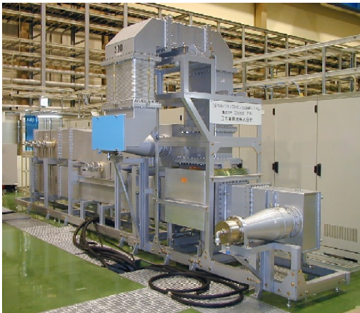
324MHz 3MWpeak WR-2300 Waveguide Circuit Combined with Circulator, Dummy Load, 3dB Hybrid Divider, RF monitor, Phase Shifter, etc...
